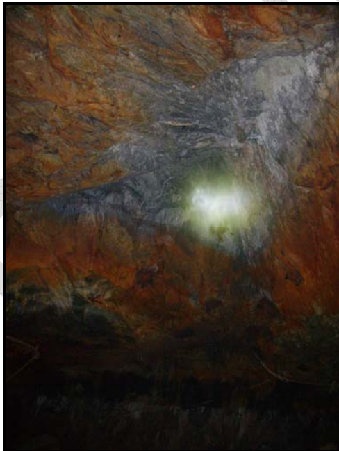
Figure 8.1 Wedge Failure Close to Pump Station
